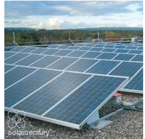
Figure 1. Framed PV modules
