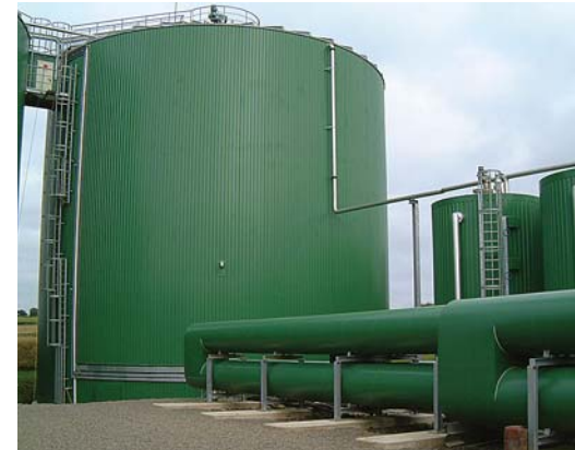
Photo 1. Holsworthy Biogas Plant
